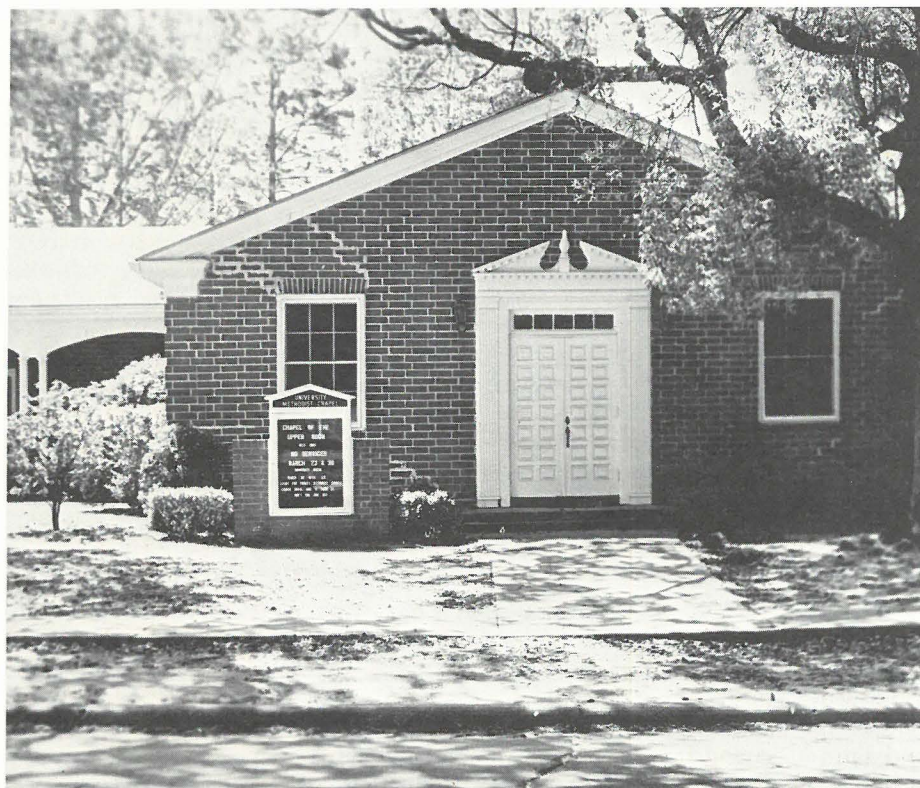
The original chapel of the Jefferson Street student house shows effects of pipe clay on its foundations.
